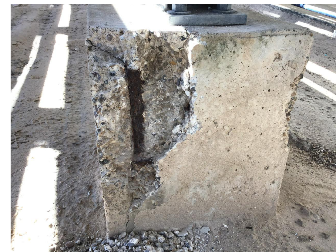
Figure 2. Typical 18" square pedestal cracking. Same pedestal as below
