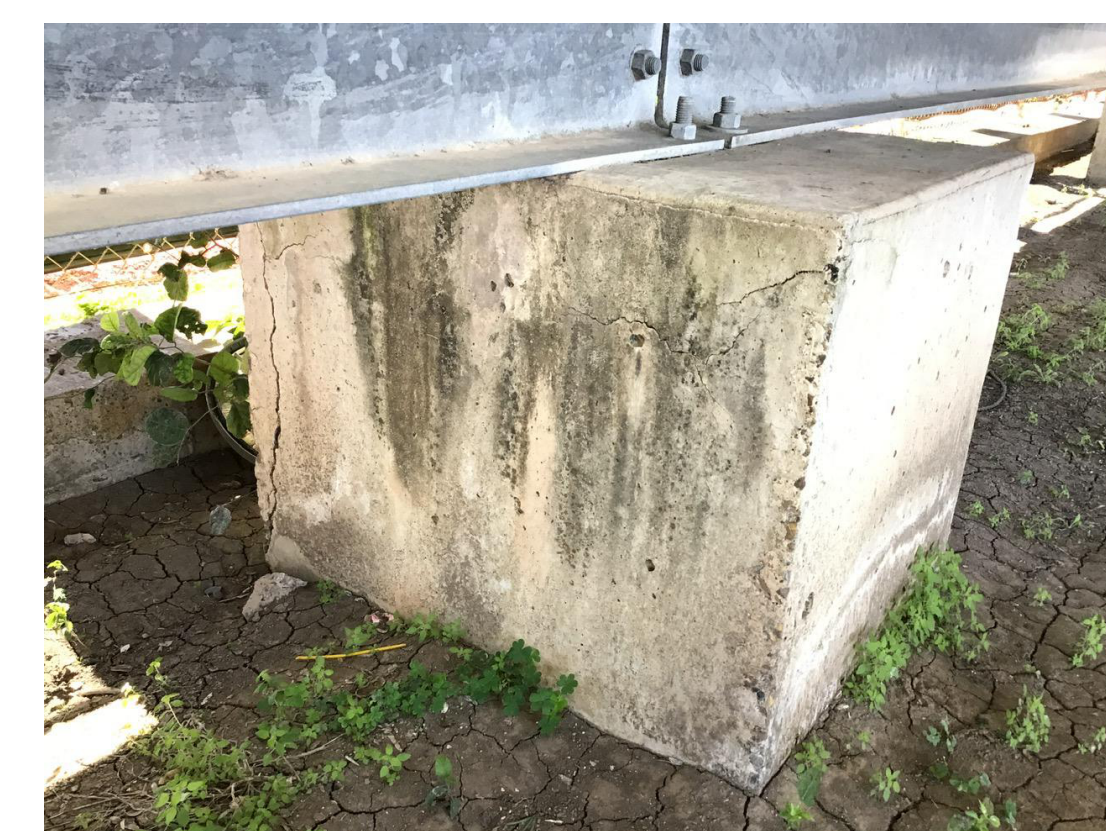
Figure 3. Typical 24" x 32" pedestal cracking
