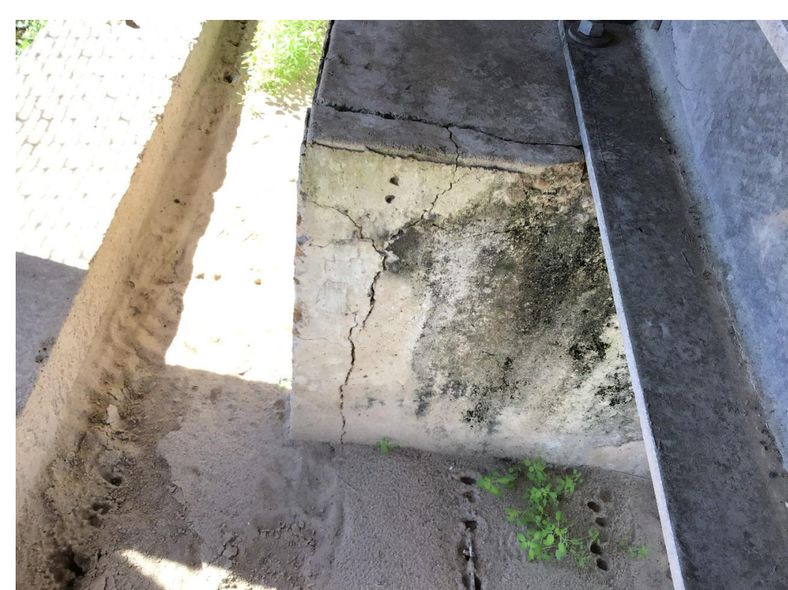
Figure 1. Typical 18" square pedestal cracking
